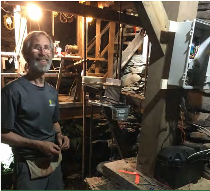
Tom Nostrand building 12 volt hydroelectric system using small Tyler turbine
